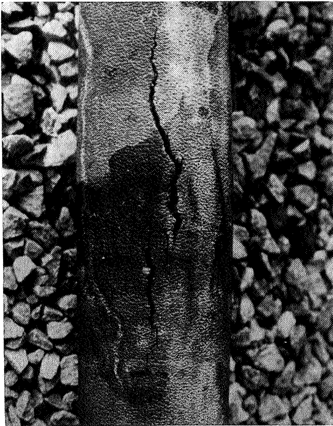
Figure 4. Longitudinal rupture in a HK-40 tube.
